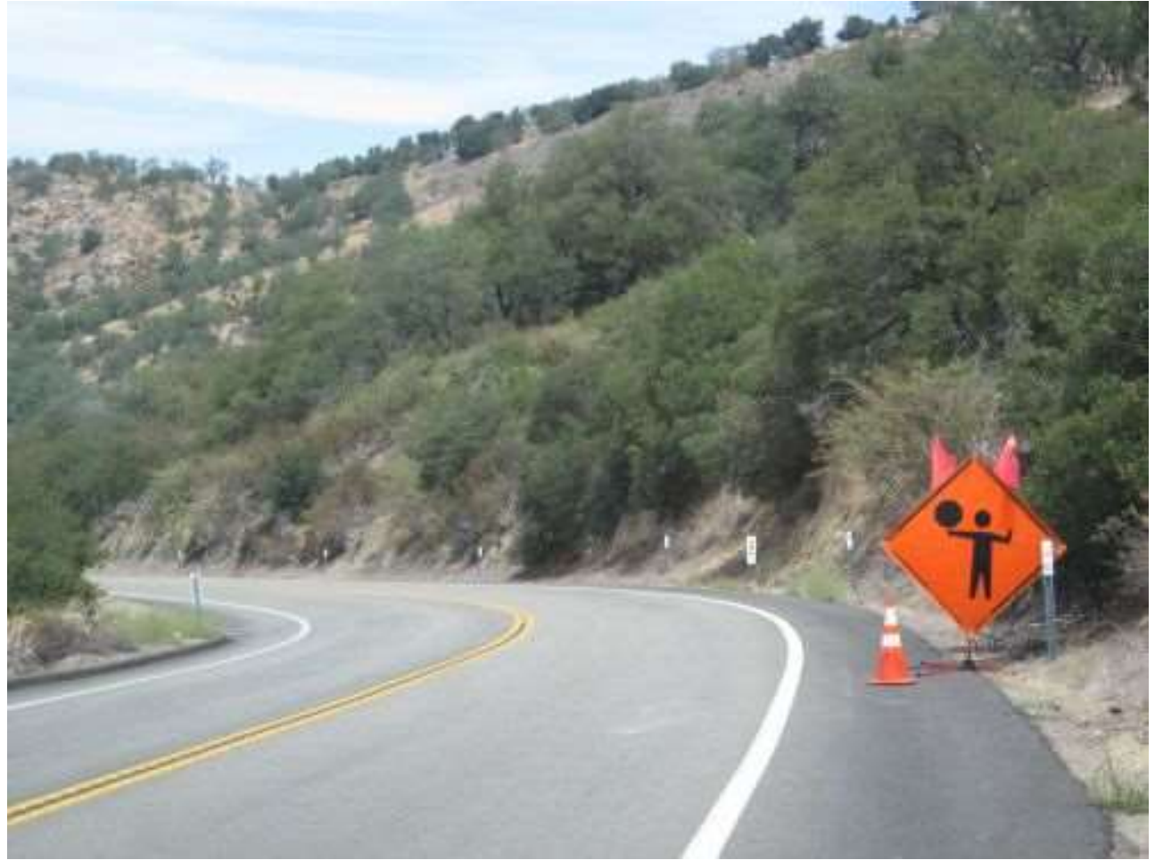
Photo 8: Traffic control measures were implemented along Old Julian Highway during wire pulling activities in accordance with APM TRA-1.
