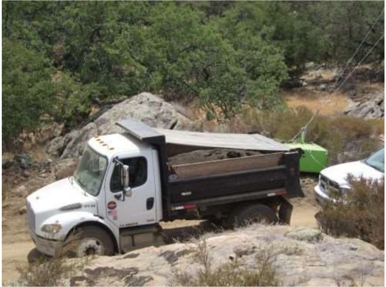
Photo 3: Loads of spoil and construction waste debris were observed covered when hauled off site in order to prevent sediment transport.
