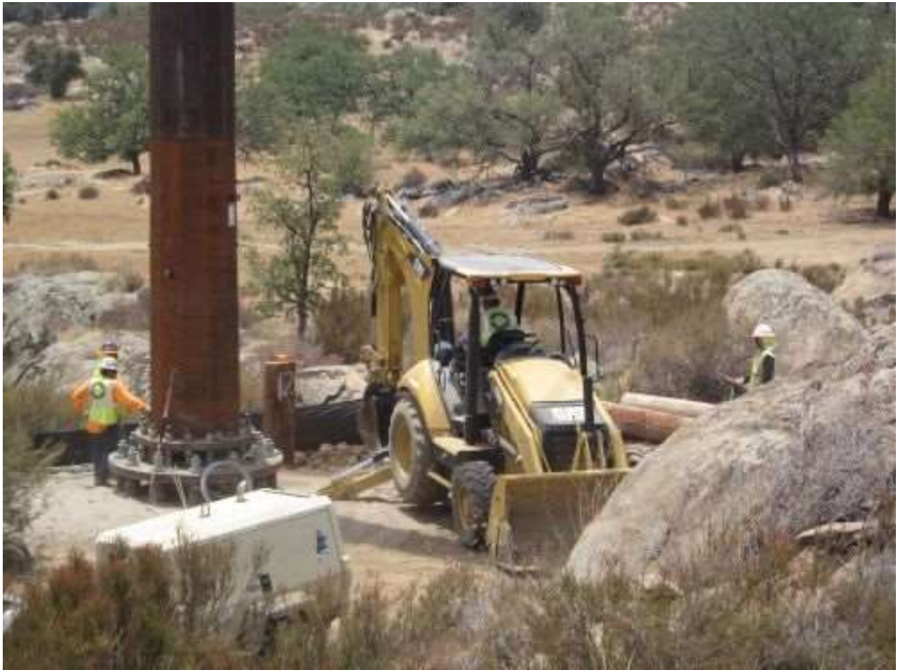
Photo 2: Crews were observed removing pole butts at Location 123 and hauling materials off site.
