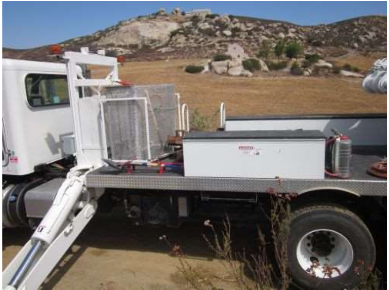
Photo 6: Fire tools (a shovel, a 5-gallon water pump, fire extinguisher, and pulaski) were observed staged in vehicles and “fire watch” was observed designated during overhead line work in accordance with the Project Fire Plan (APM HAZ-2).
