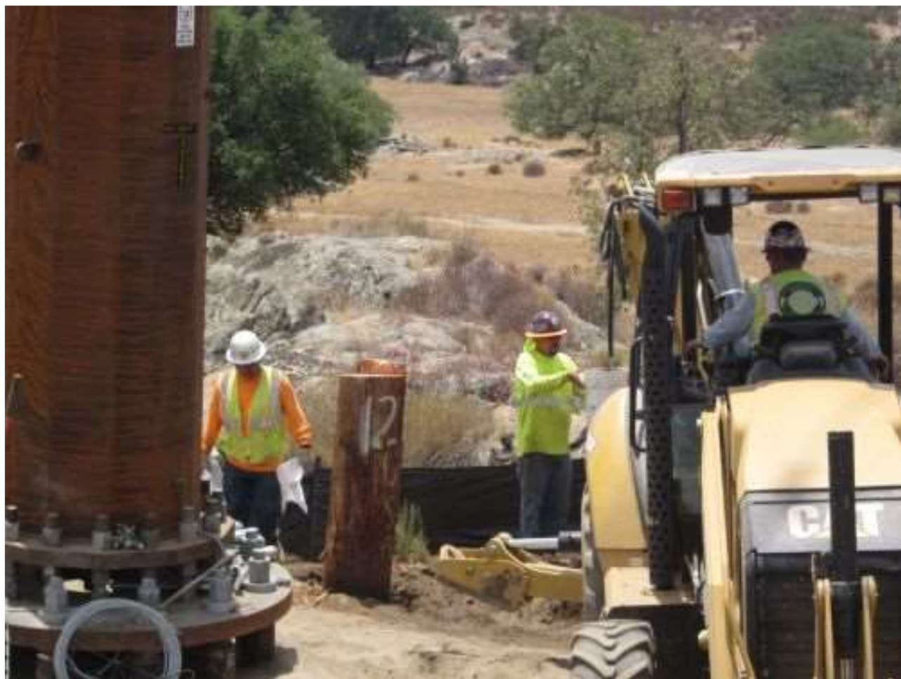
Photo 4: Crews were observed using a spill kit in accordance with MM HAZ-2 at Location 123 to clean up a hydraulic fluid leak resulting from a broken hose on a piece of equipment.
